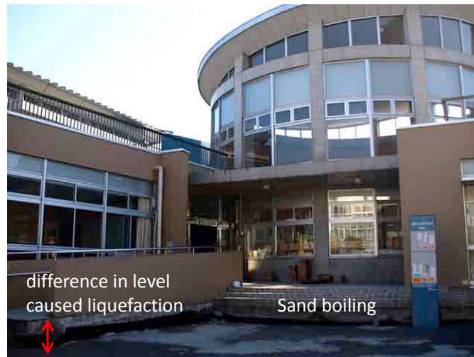
Picture 1: Liquefaction damage at Area 1
