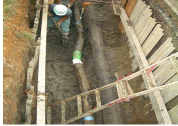
Figure 1. Upheaval buckling of 4” pipe
