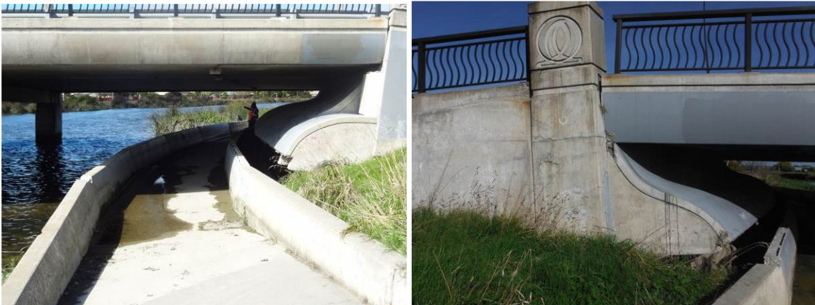
Figure 4 Rotation of south abutment from west (left) and east (right)
